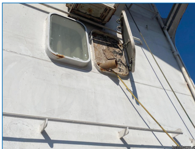
Non ship type air condition hose passing through cabin window on starboard side.
